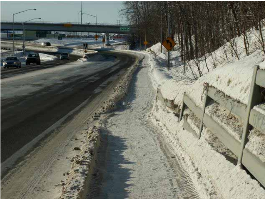
Here is the existing retaining wall cutting into the sidewalk opposite the AKRR Engine Shop.
